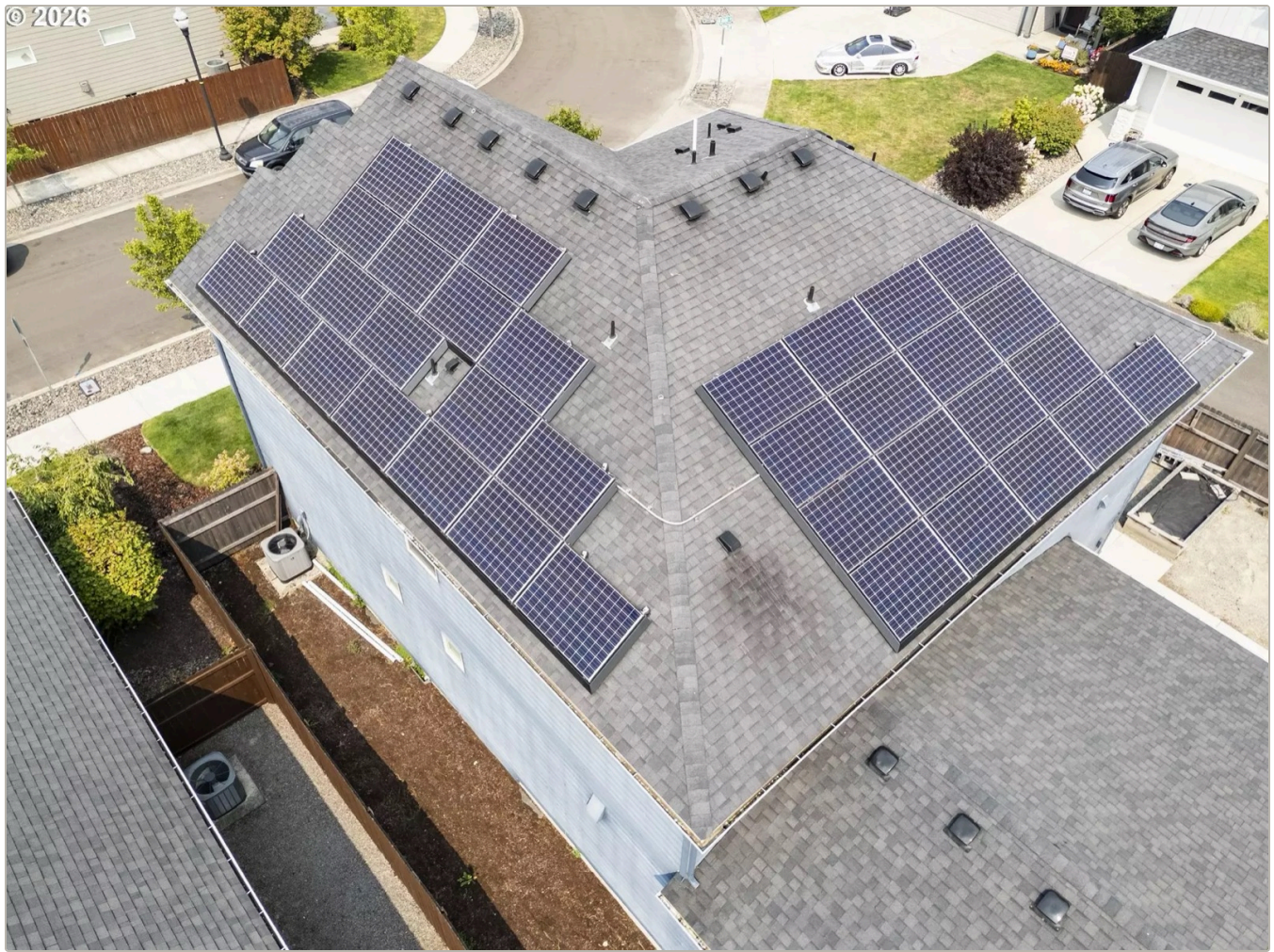
FIG. 02 — The array from directly above — the full run of modules across both roof planes. The grey unit on the pad against the wall at lower left is the AC condenser, not part of the solar system.
