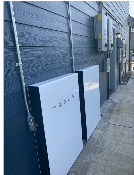
FIG. 01 — The two Tesla Powerwalls on the garage's north wall, at the rear end of the north side yard. The grey boxes above them are the solar inverters.
